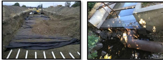
Figure 11. Anspach site under construction in 2012 (left) and new intake structure in 2015 (right).
