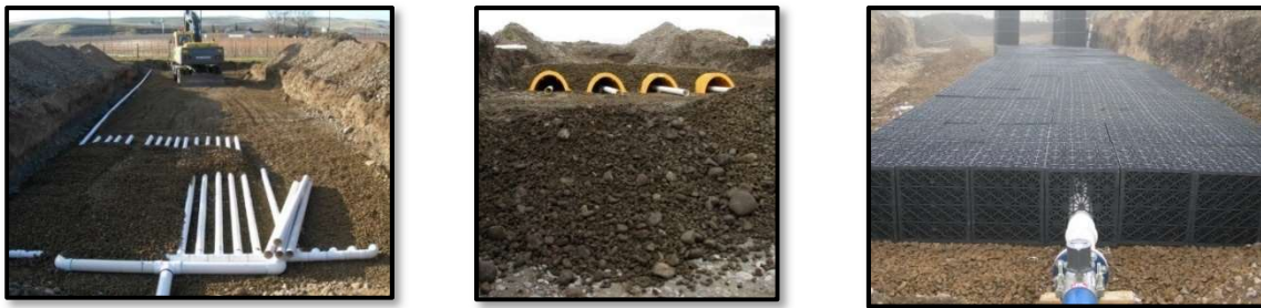
Figure 18. Infiltration galleries #2 (left), #3 (center), and #4 (right) being installed at the Johnson site.
