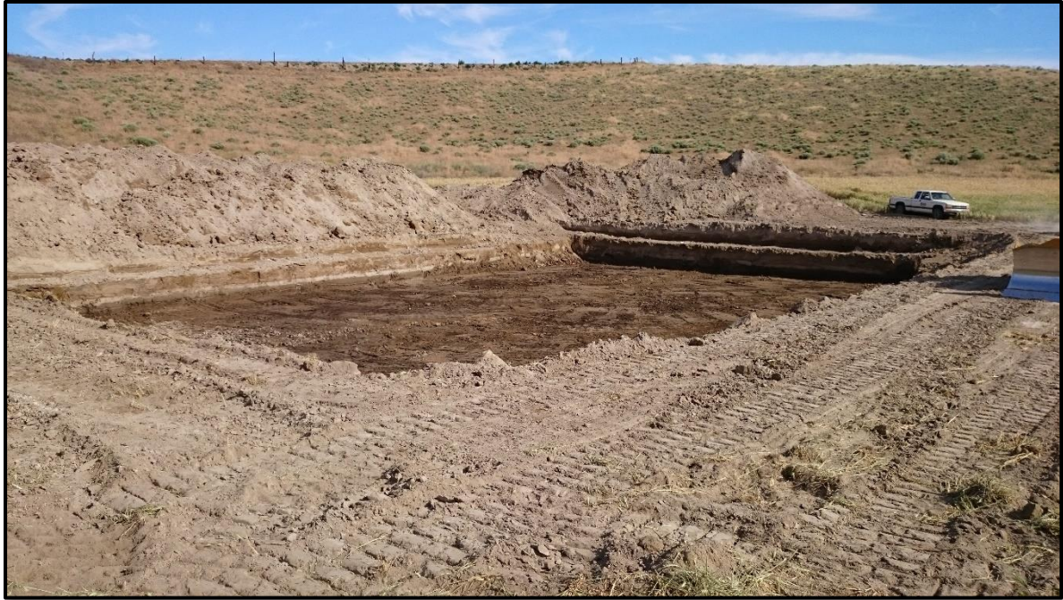
Figure 17 - Infiltration gallery area for the Last Chance Road Aquifer Recharge site.
