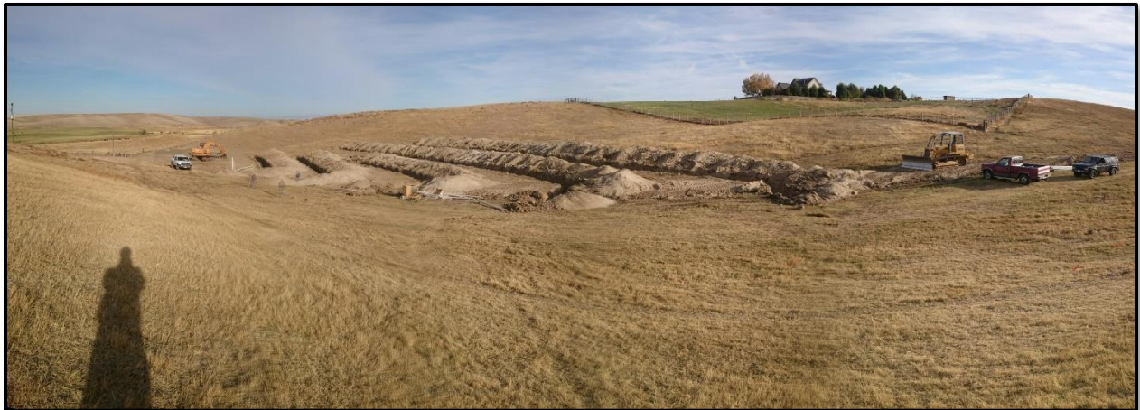
Figure 19 - Photo of the WA Mud Creek Aquifer Recharge site under construction. The photo shows the excavated trenches for the infiltration gallery on the south side of Mud Creek.
