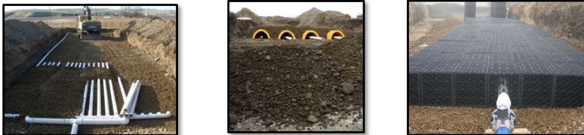
Figure 16 - Photographs of infiltration galleries #2 (left), #3 (center), and #4 (right) being installed at the Johnson site.
