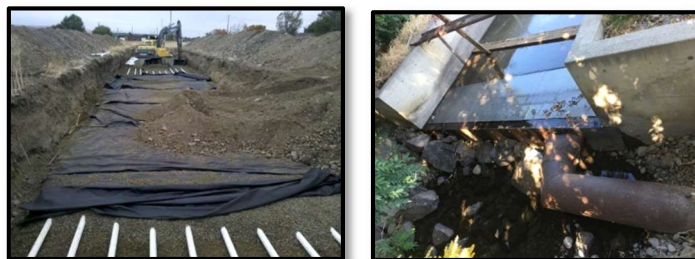
Figure 10 - The Anspach site during construction in 2012 (left) and new intake structure in 2015 (right).
