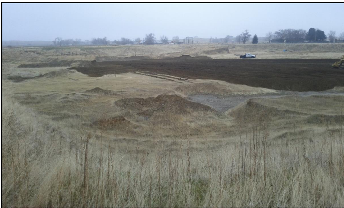
Figure 12 - Photo during expansion of the Locher Road site's main recharge basin, December 2011.
