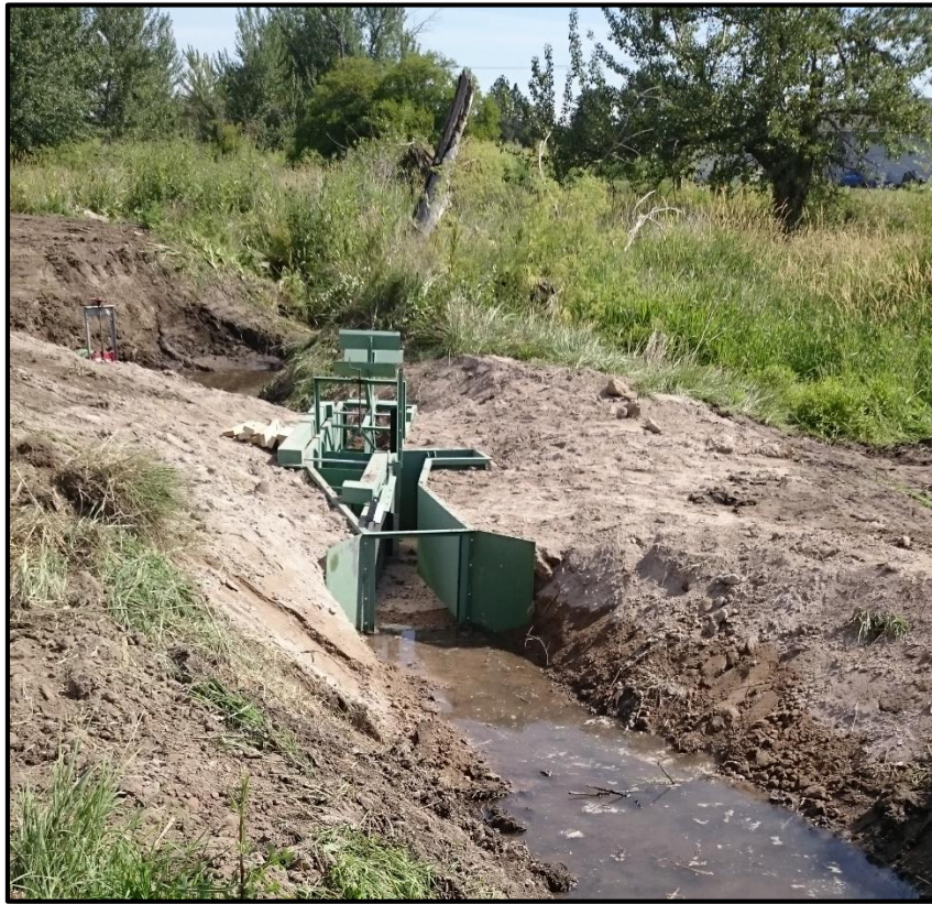
Figure 18 - Irrigation ditch, fish screen and intake (back left) for the Last Chance Road Aquifer Recharge site.
