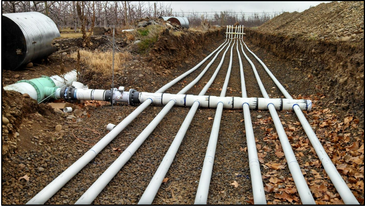
Figure 12 - Turn out structure, valve, flow meter and pipe manifold for the Barrett Aquifer Recharge site. See Appendix C for design details.
