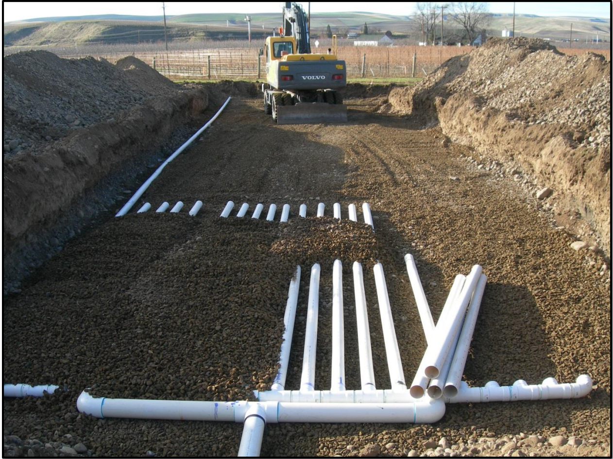
Figure 15 - Photograph of infiltration gallery #2 (IG2) being installed at the Johnson Aquifer Recharge site. IG2 is 4-inch perforated drain field pipe installed over washed gravel and buried in ~1 foot of washed gravel with geo-textile fabric on top of the gravel. See Appendix C for designs.
