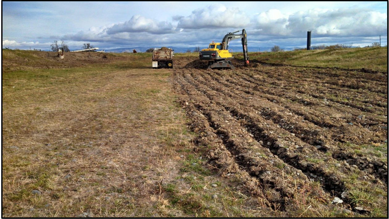
Figure 18 - NW Umapine Aquifer Recharge site during excavation and shaping of the infiltration basin. See Appendix C for design details.
