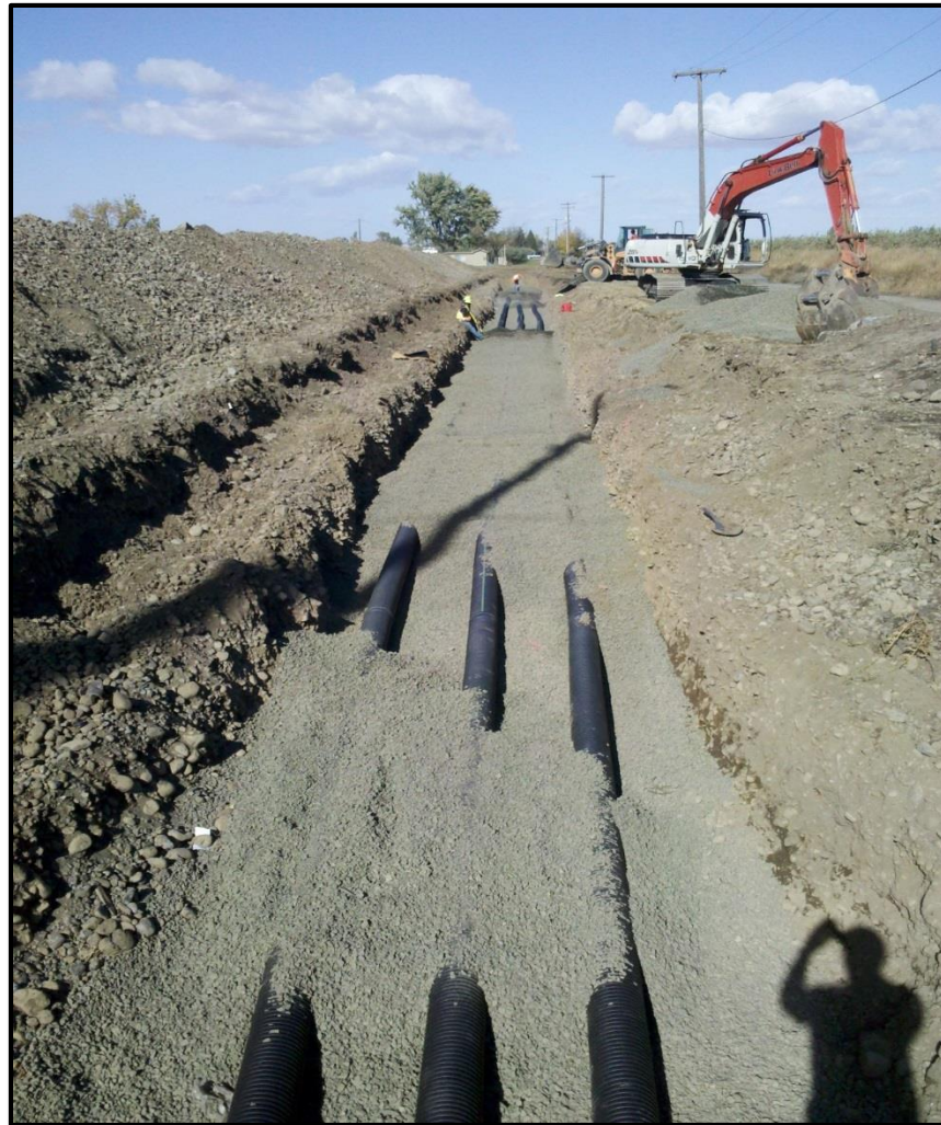
Figure 20 - The Trumbull Aquifer Recharge site under construction in October 2012. The site is approximately 300 feet long with three 8-inch pipes running the entire length. See Appendix C for design details.
