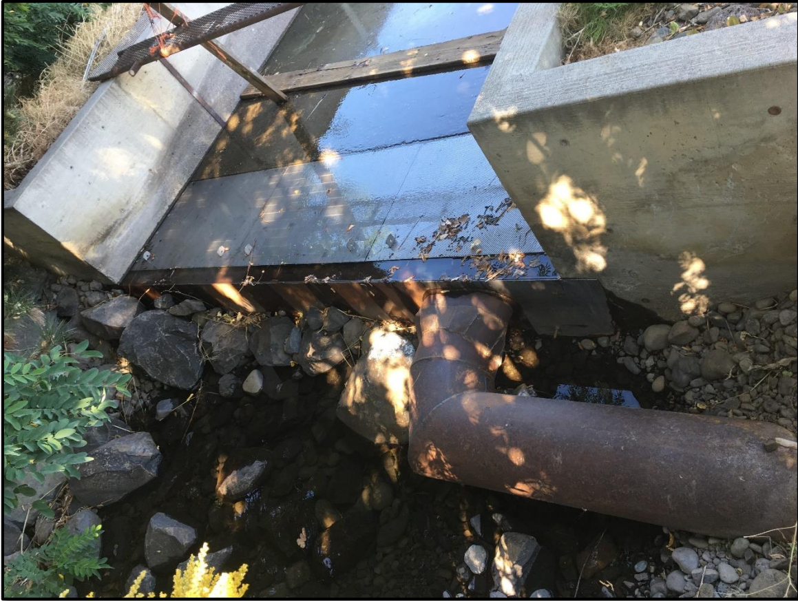
Figure 11 - New intake structure and pipeline for the Anspach AR site built in the fall/winter of 2015.
