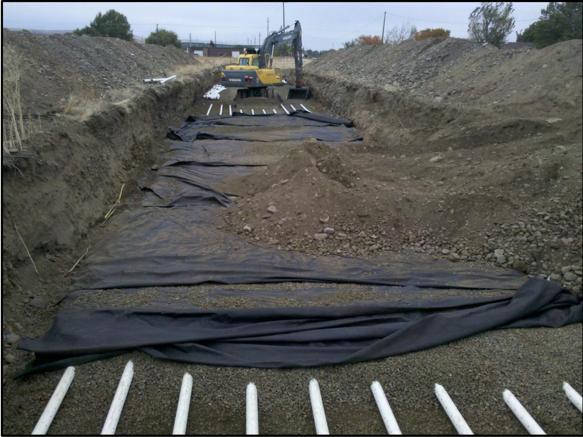
Figure 10 - The Anspach Aquifer Recharge site during construction in October 2012. This recharge site utilizes ten 4-inch perforated pipes that run approximately 200 feet. See Appendix C for designs.
