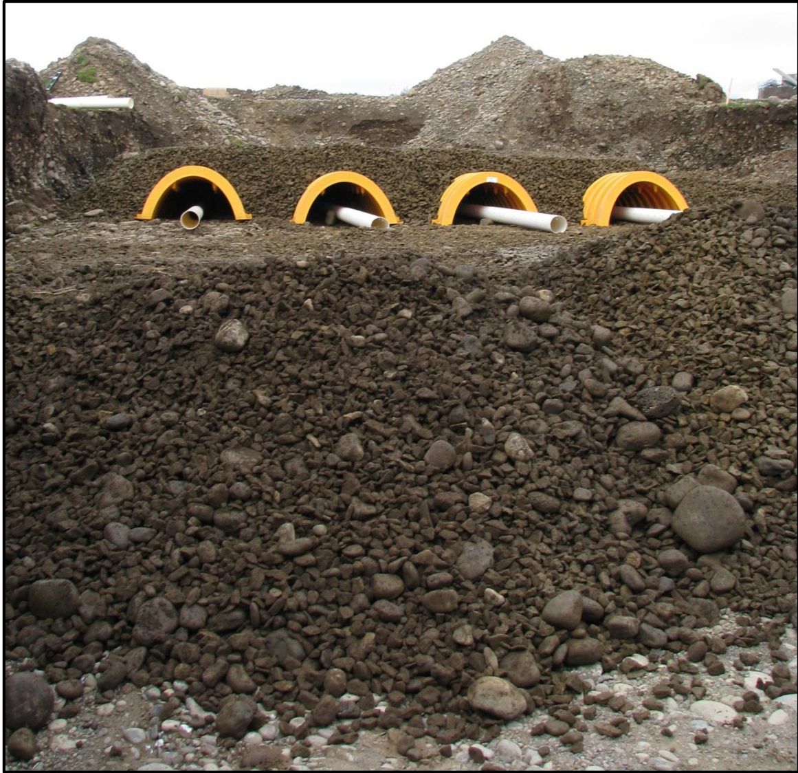
Figure 16 - Photograph of infiltration gallery #3 (IG3) at the Johnson Aquifer Recharge site. IG3 is 4-inch perforated drain field pipe installed within Stormtech stormwater chambers (yellow covers) over washed gravel and buried in ~2 foot of washed gravel with geo-textile fabric on top of the gravel. See Appendix C for designs.
