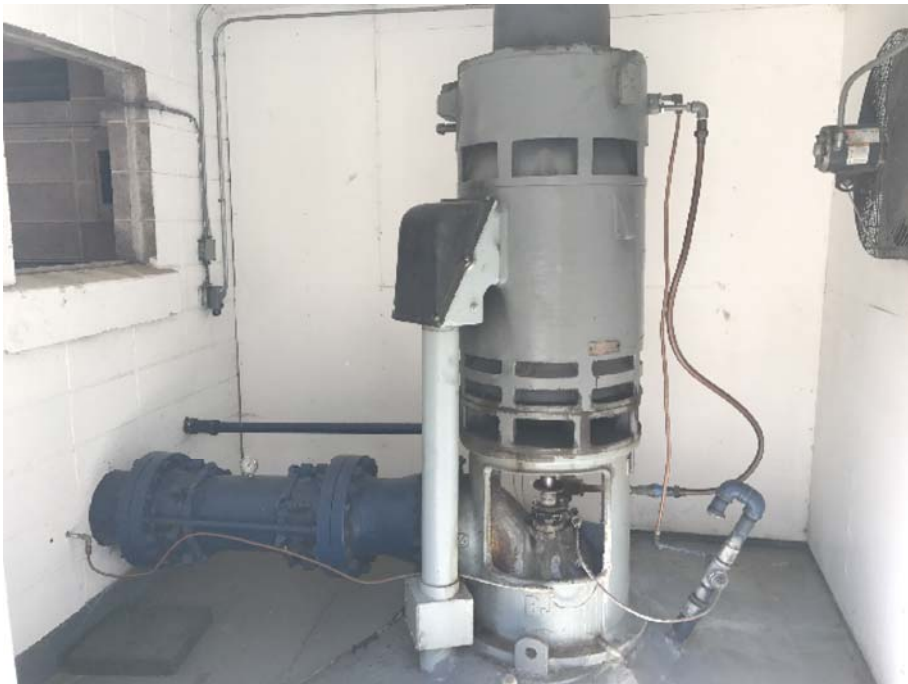
Well #8 inside south end pump
