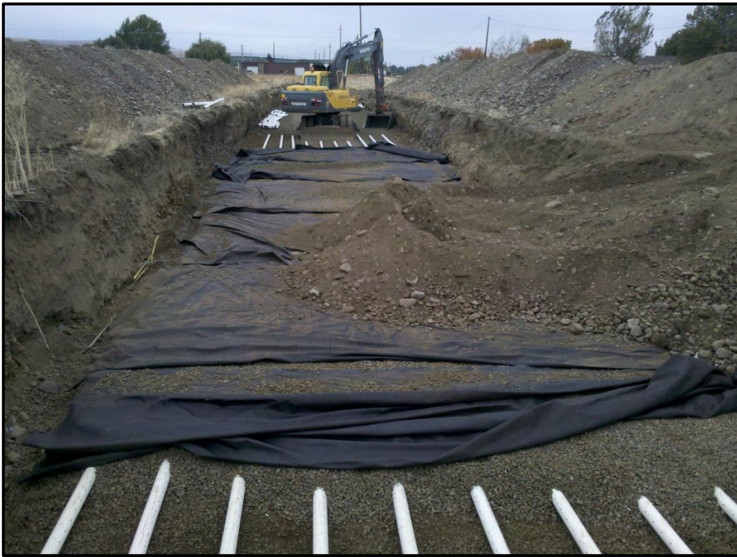
Figure 2 - Photograph of the Anspach aquifer recharge site during construction. Photo is looking west from the up-gradient end of the project.
