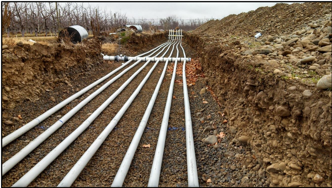
Figure 4 - Photograph of the Barrett aquifer recharge site during construction. Photo is taken near the middle of the site looking east.
