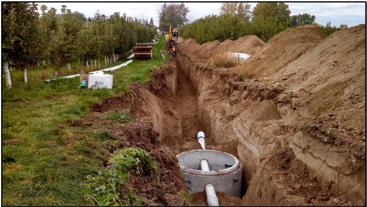
Figure 16 - Photograph of the LeFore Road aquifer recharge site during construction. Photo was taken near the up-gradient end of the project looking west.
