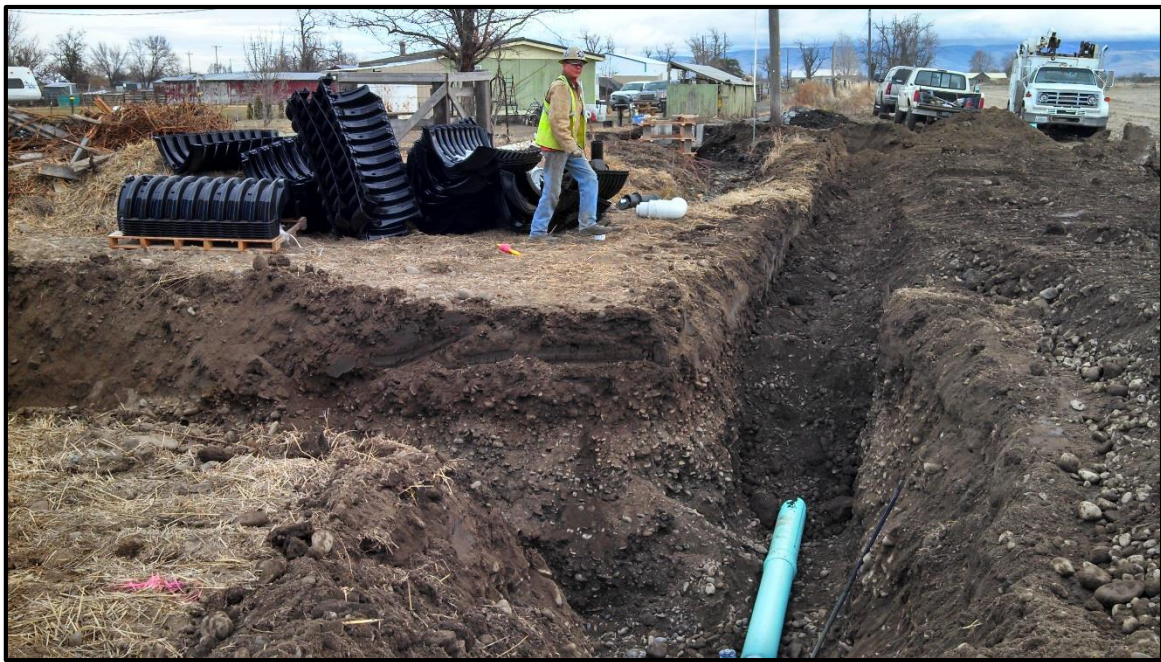
Figure 28 - Photograph of the West Ringer Road aquifer recharge site during construction. Photo was taken near the middle of the site looking east.
