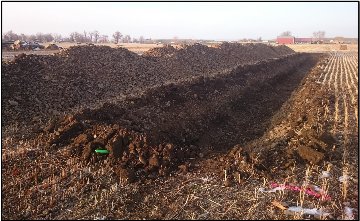
Figure 11 - Photograph of the Fruitvale aquifer recharge site during construction. Photo is taken near the southern end of one of the infiltration gallery looking north.
