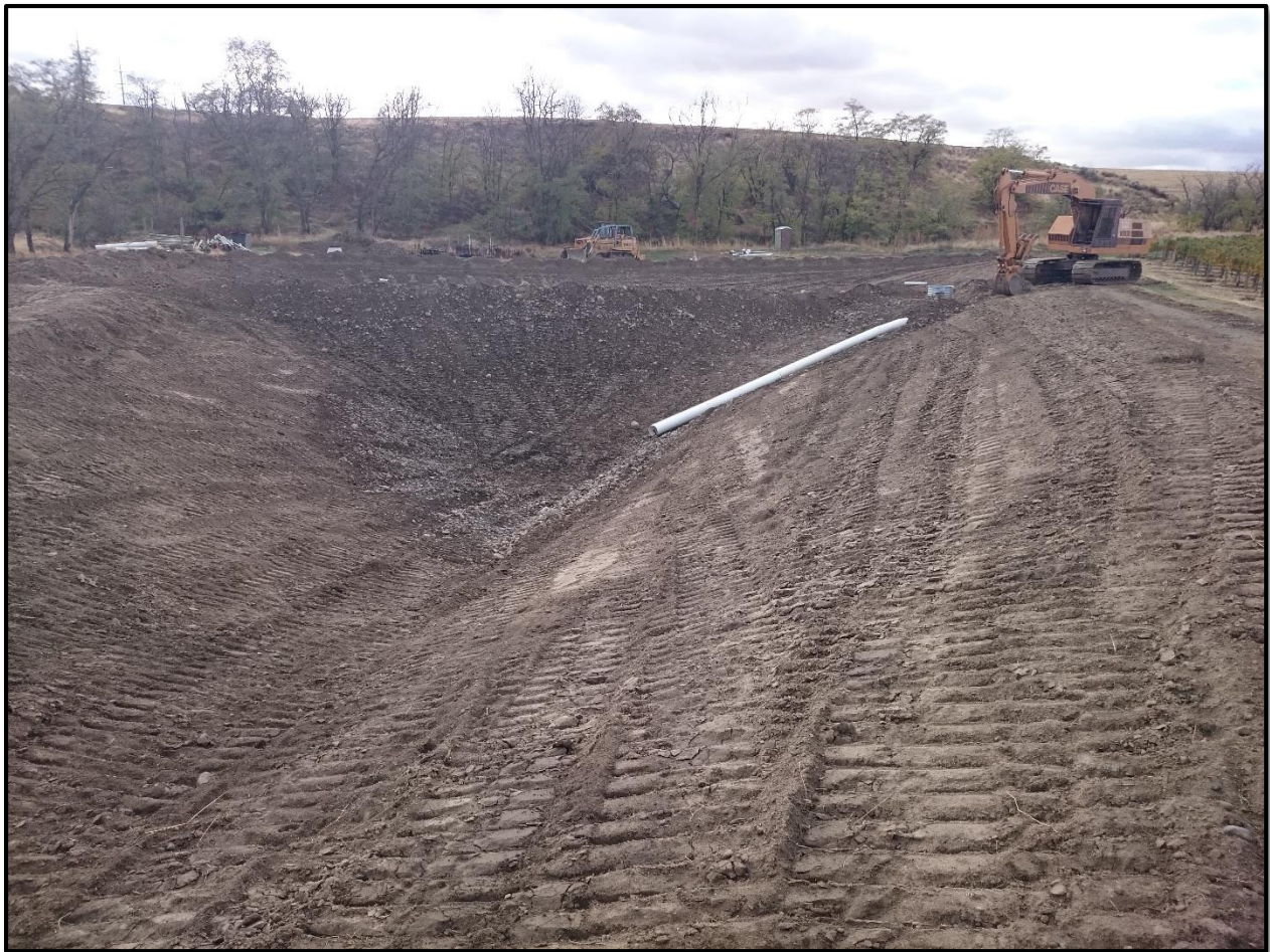
Figure 6 - Photograph of the Chuckhole aquifer recharge site during construction. Photo is taken at the north end of the project looking south.
