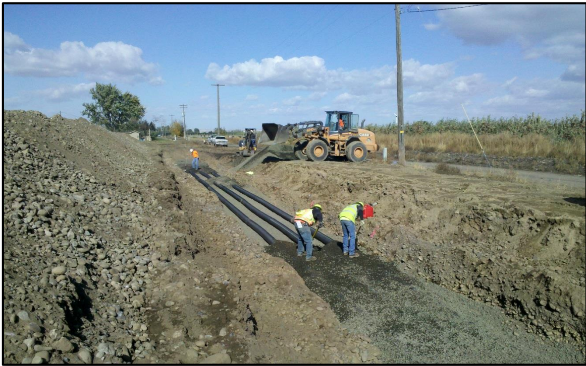
Figure 26 - Photograph of the Trumbull aquifer recharge site during construction. Photo is looking north from the up-gradient end of the project.
