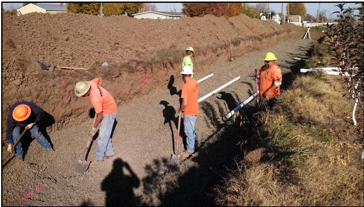
Figure 9 - Photograph of the East Trolley Lane aquifer recharge site during construction. Photo is taken near the northern end of the project looking northwest.
