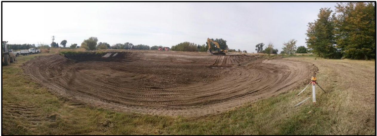
Figure 19 - Photograph of the Mud Creek aquifer recharge site during construction. Photo is taken from the east side of the project looking west.
